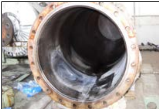
Damaged heat exchanger
